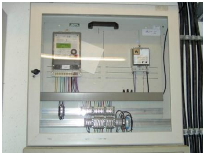
Converter with decoupling relays
